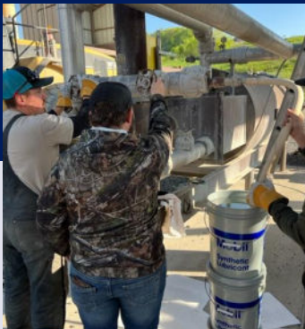
FIGURE 5: MOBIL SOLVANCER BEING ADDED TO THE HTS
